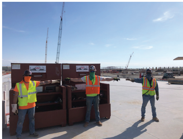
Union ironworkers working for steel erector National Steel City are maintaining social distancing using Proximity Trace at the $1.9-billion Kansas City International single-terminal project. Photo courtesy of National Steel City
